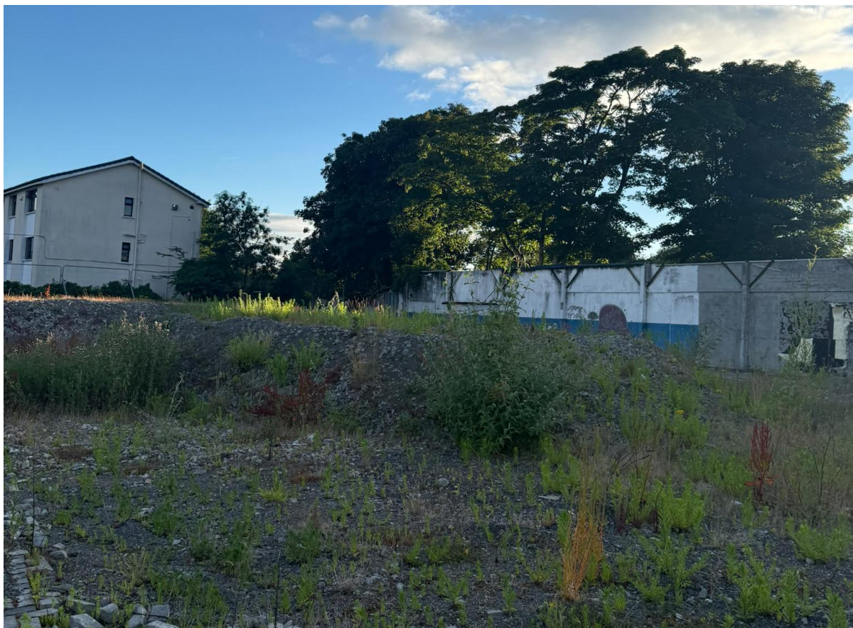
Plate 3. Rubble pile on site
